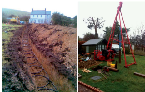
Fig. 6 The installation of ground loops for GSHP systems using slinky horizontal pipes (left) and a vertical borehole (right). source: Staffell et al, 2012
